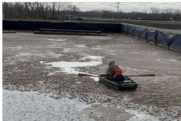
Staff adjusting the SBR Decant Header
