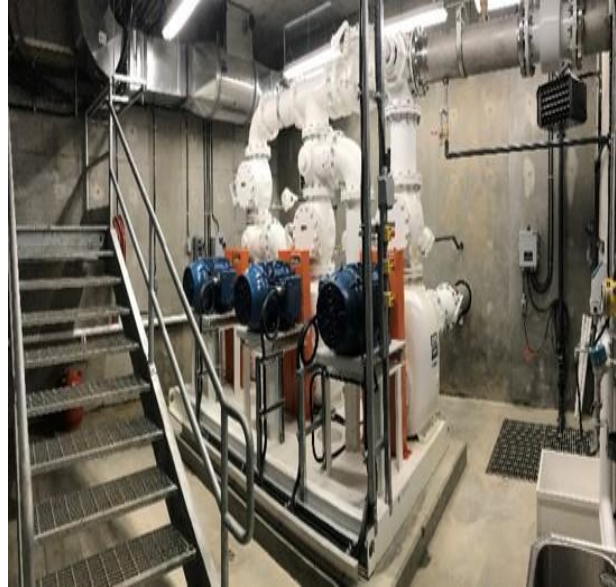
Poplar Bluff Lift Station- Interior
