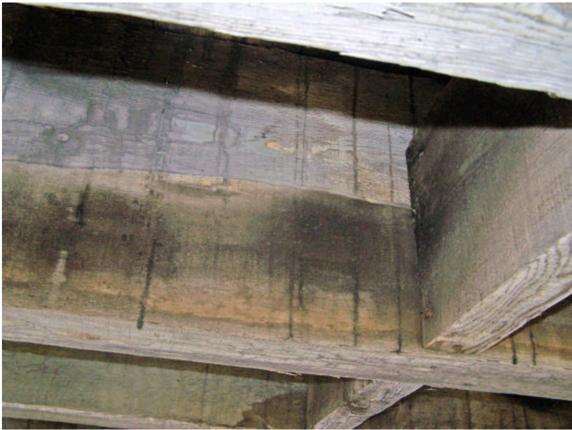
Photo 25 – Stringer (severe splitting)
