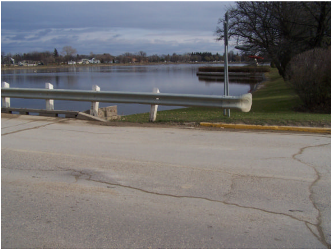
Photo 33 – Guardrail post missing
