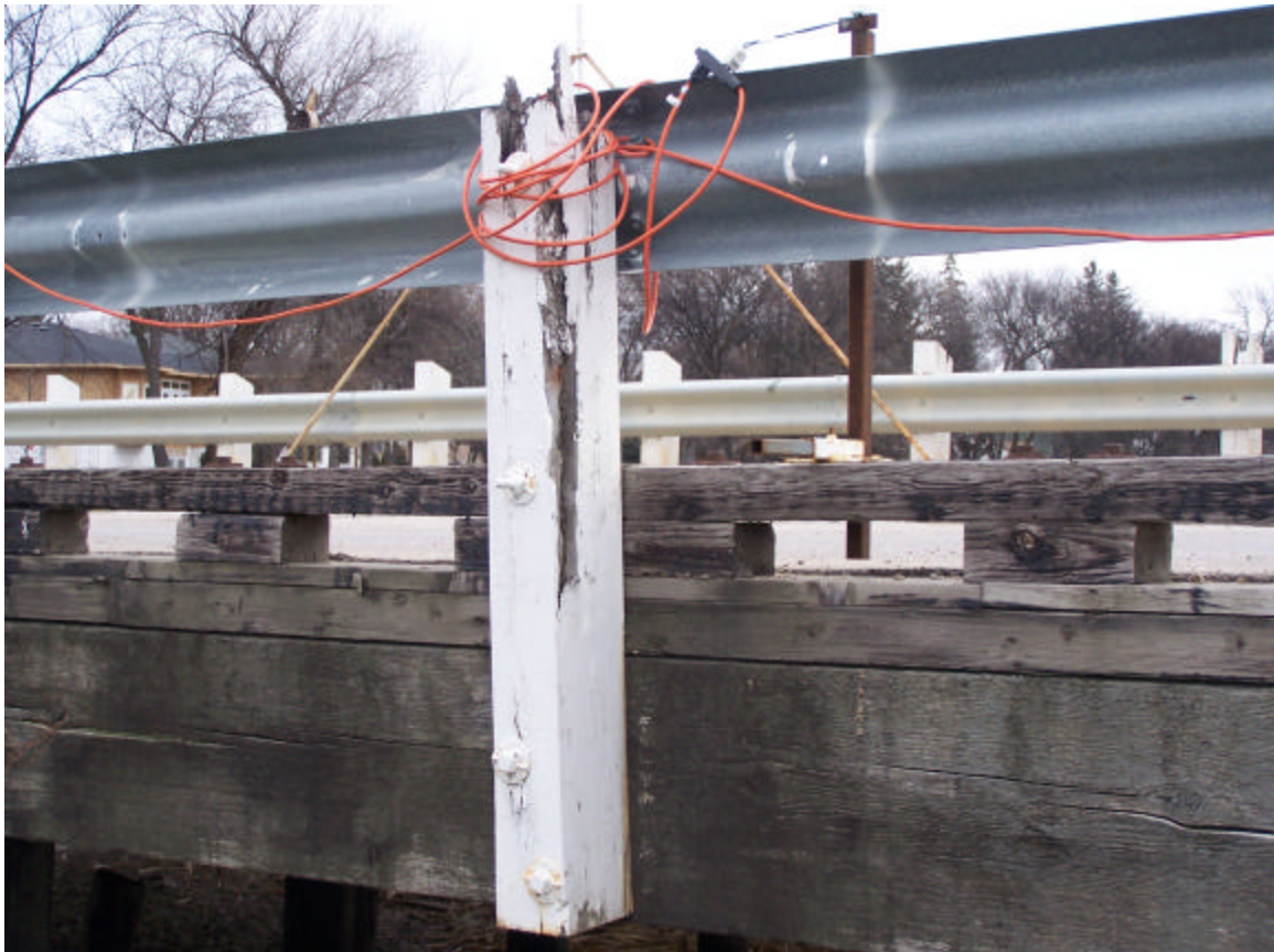
Photo 28 – Handrail post damage
