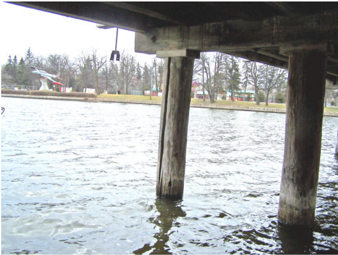
Photo 11 – Pile (severe splitting)
