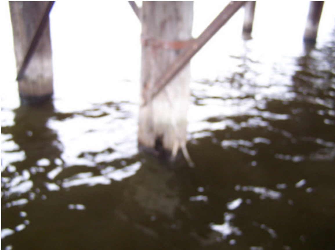
Photo 12 – Pile (partial splitting)
