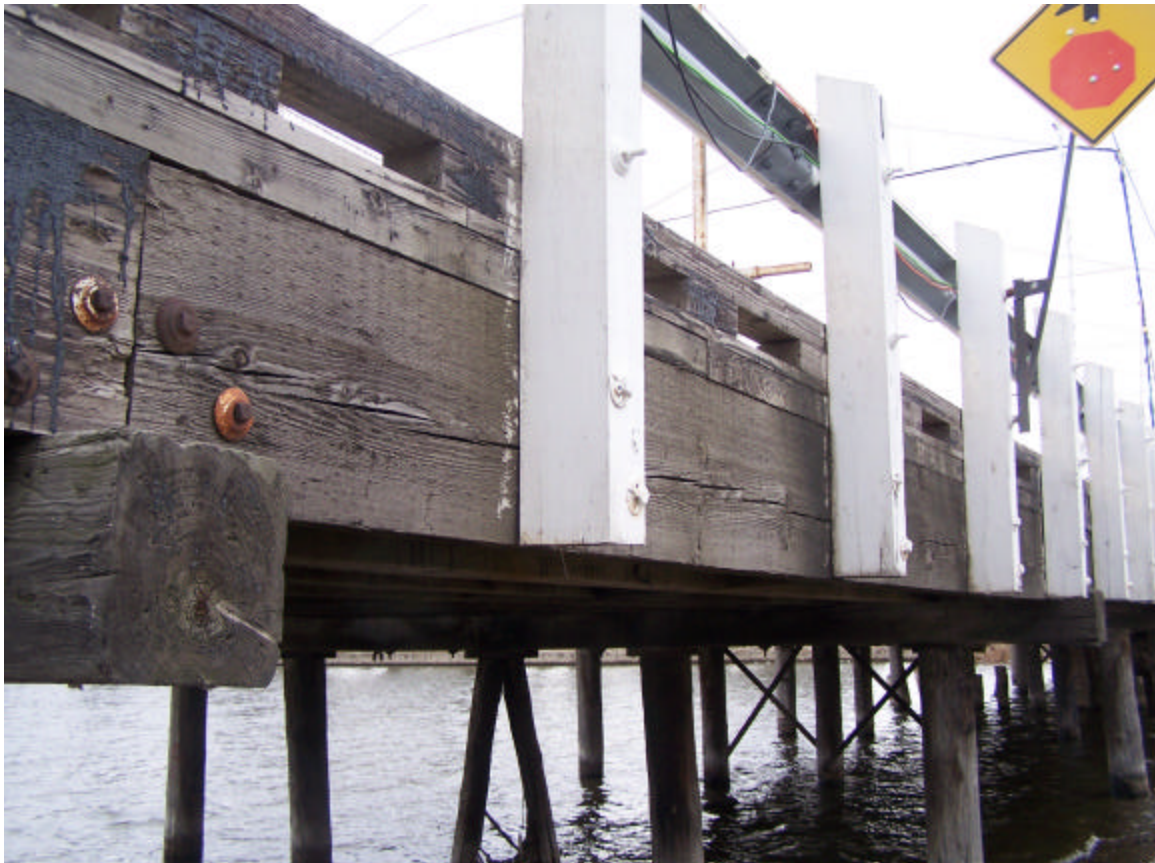
Photo 22 – Stringer (severe splitting)
