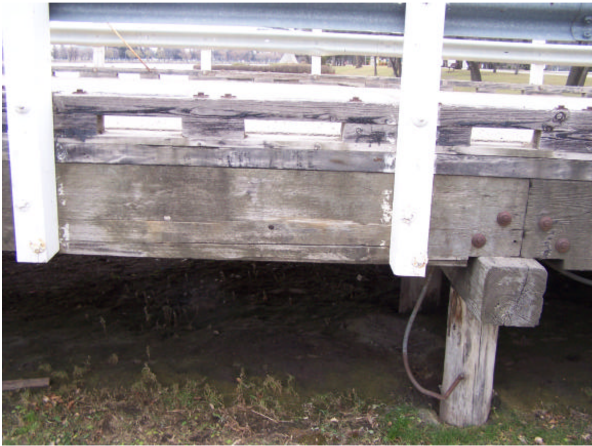
Photo 17 – Stringer (minor splitting)
