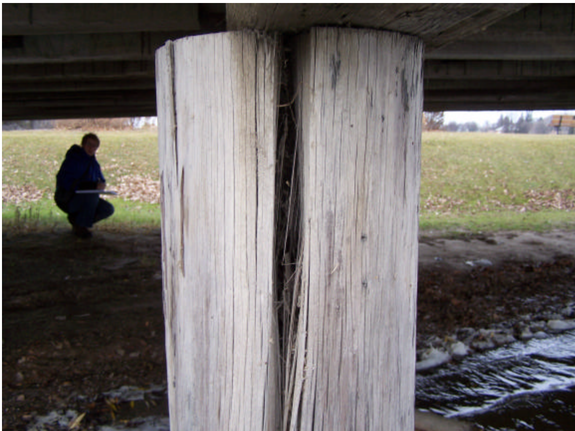
Photo 2 – Pile (severe splitting)
