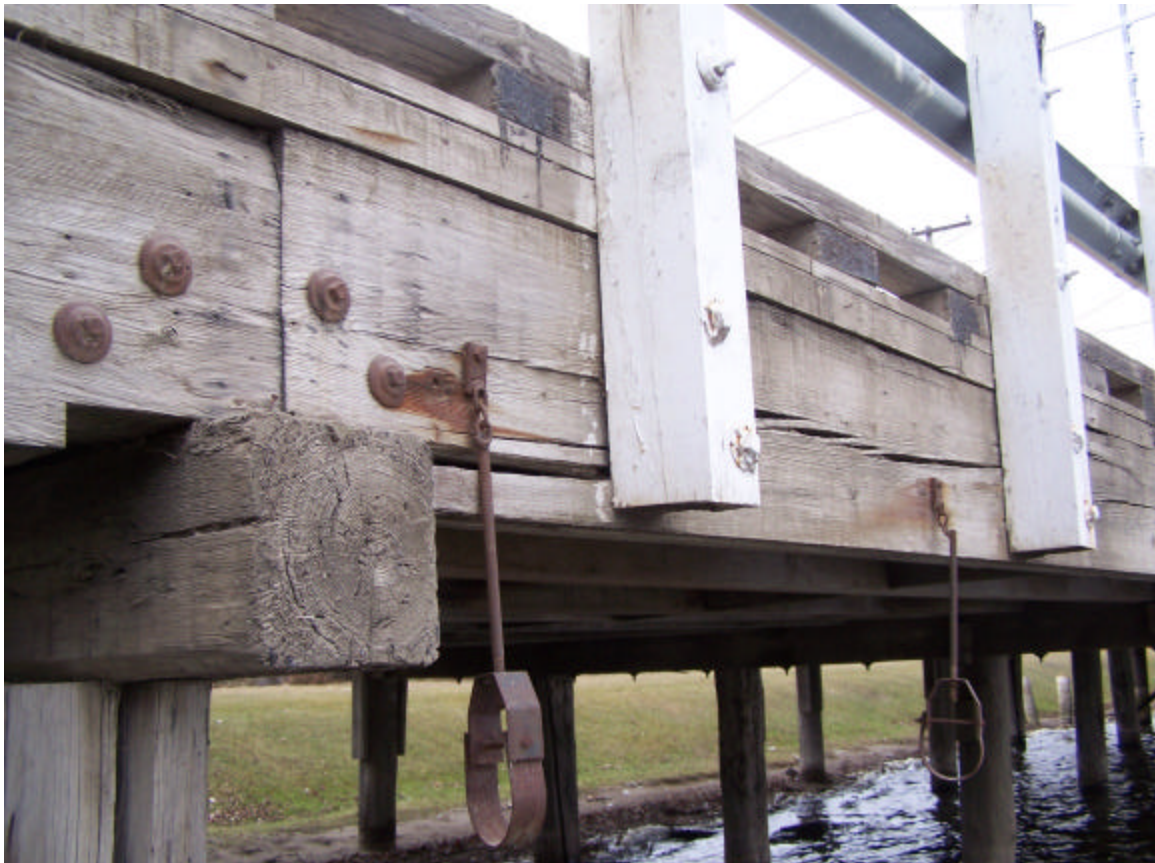
Photo 18 – Stringer (severe splitting)
