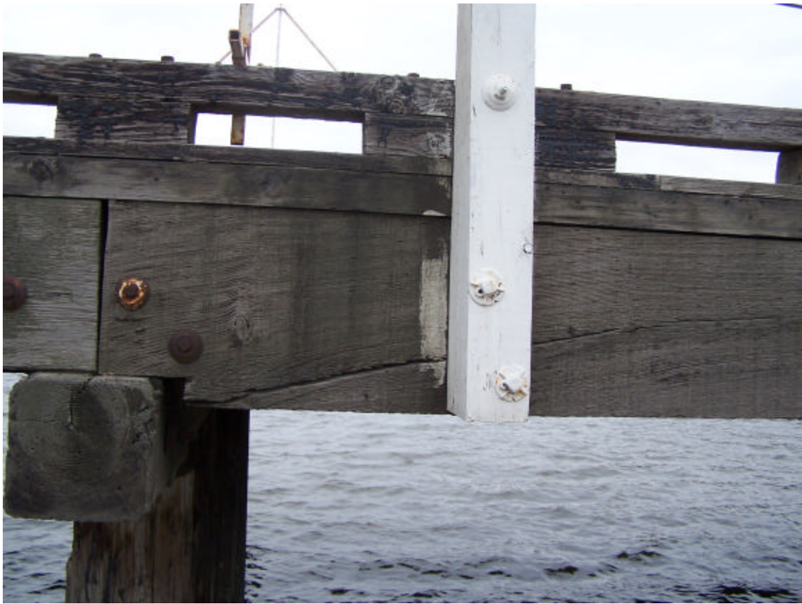
Photo 21 – Stringer (severe splitting)
