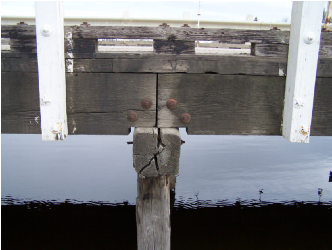
Photo 15 – Pile cap (severe splitting)
