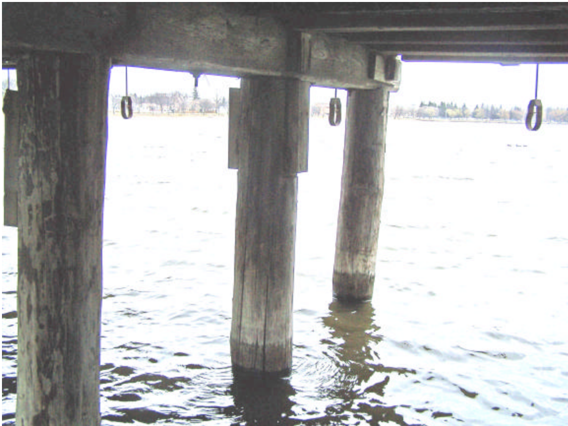
Photo 4 – Pile (partial splitting)
