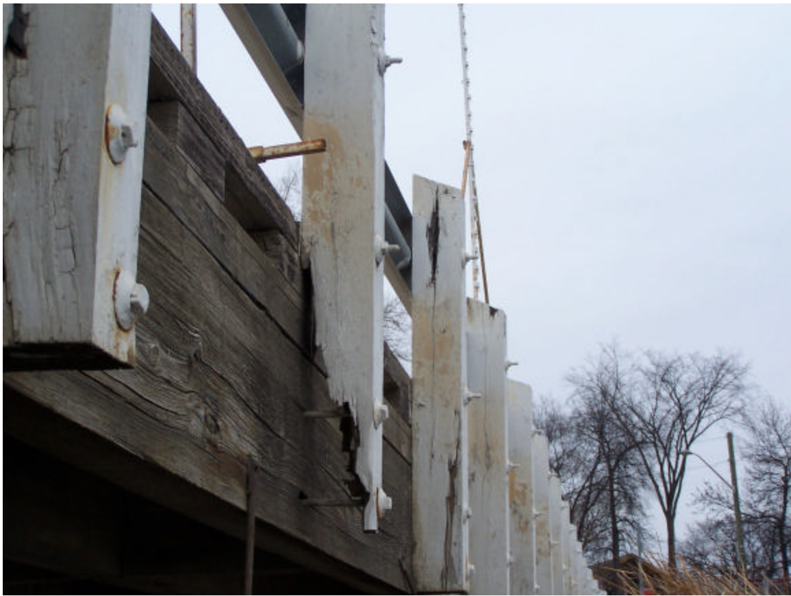
Photo 29 – Handrail post damage
