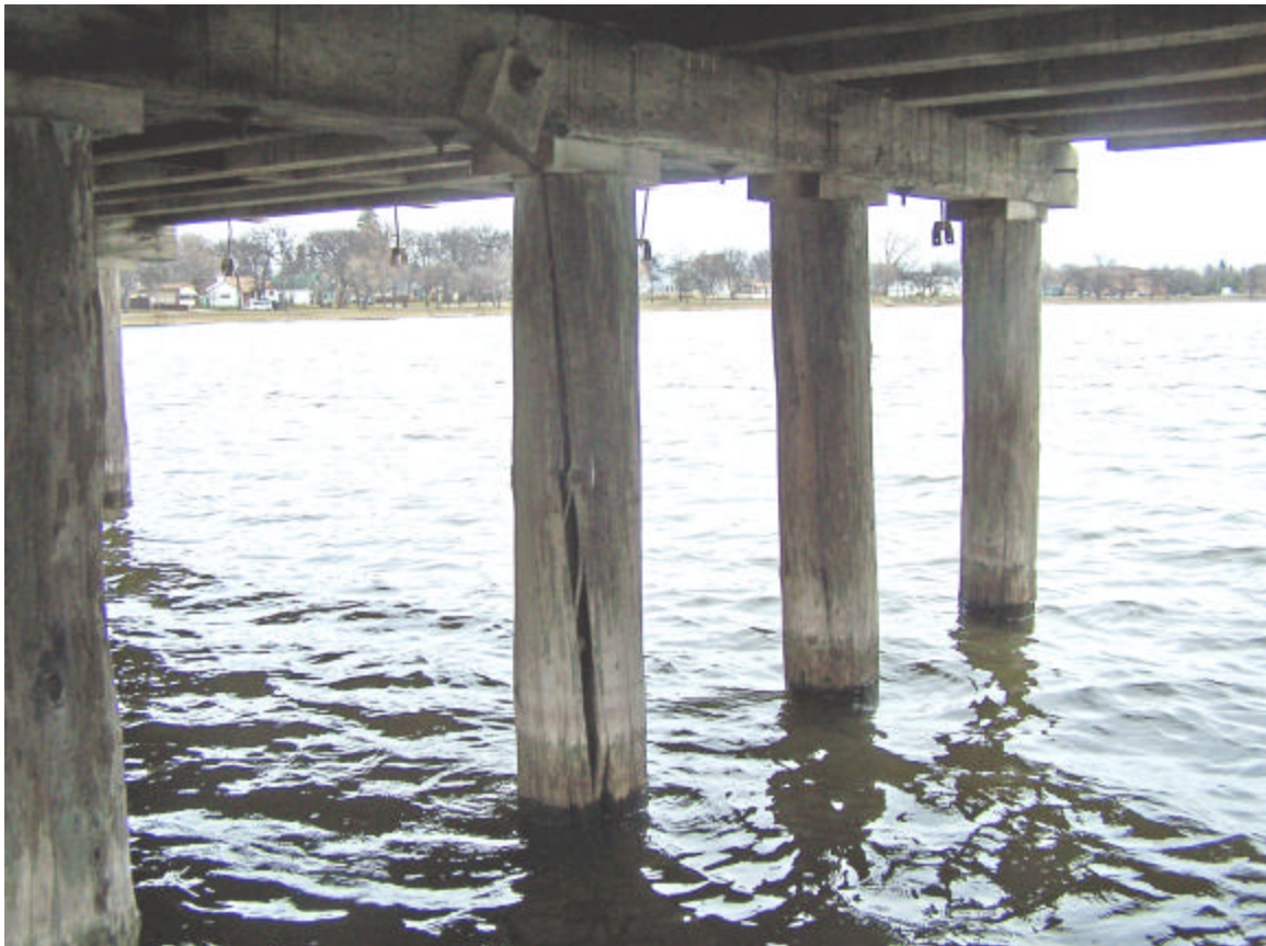
Photo 10 – Pile (severe splitting)
