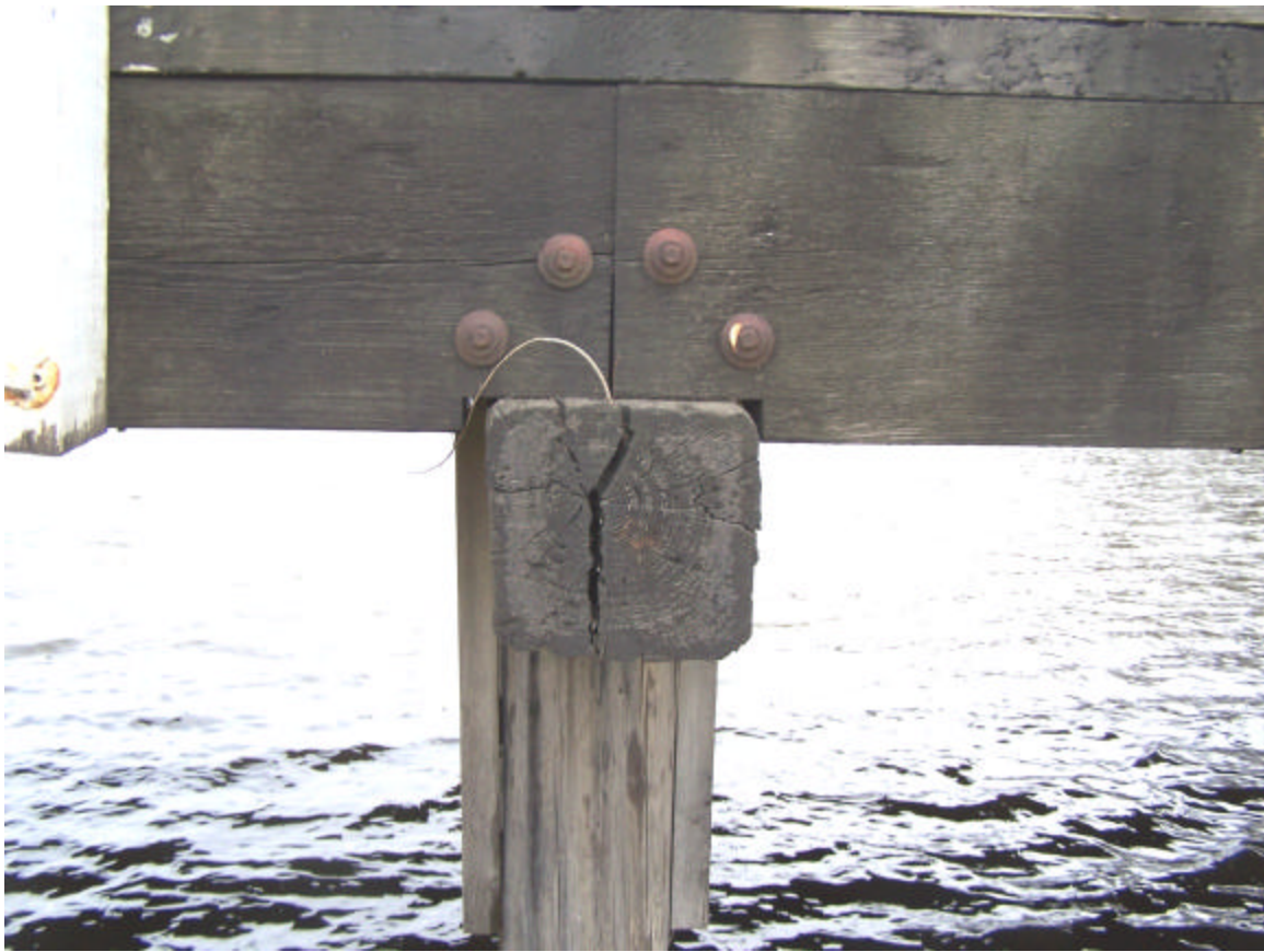
Photo 13 – Pile cap (minor splitting)
