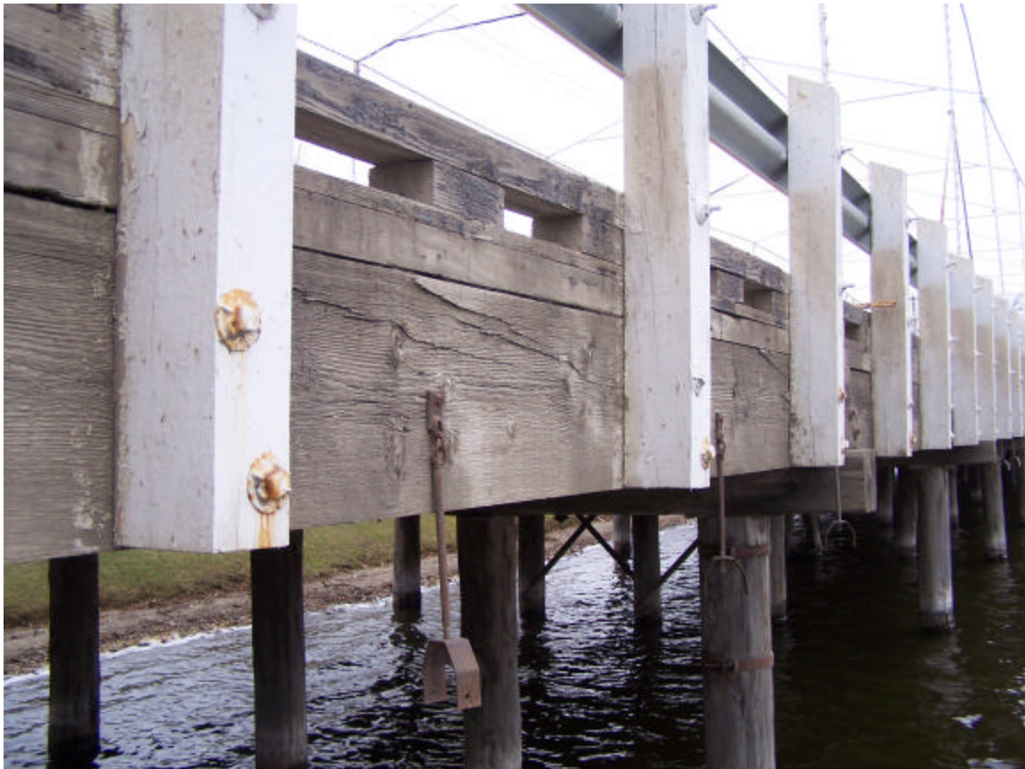
Photo 20 – Stringer (minor splitting)
