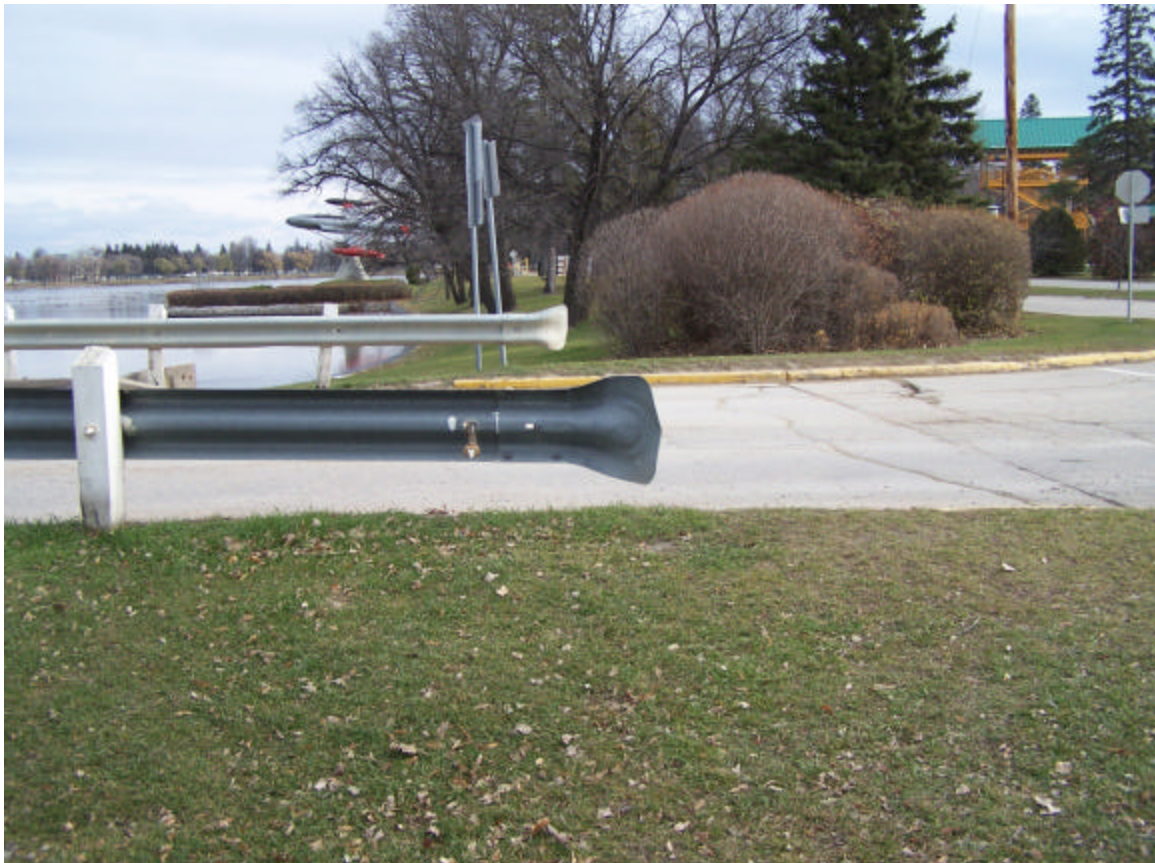
Photo 34 – Guardrail post missing
