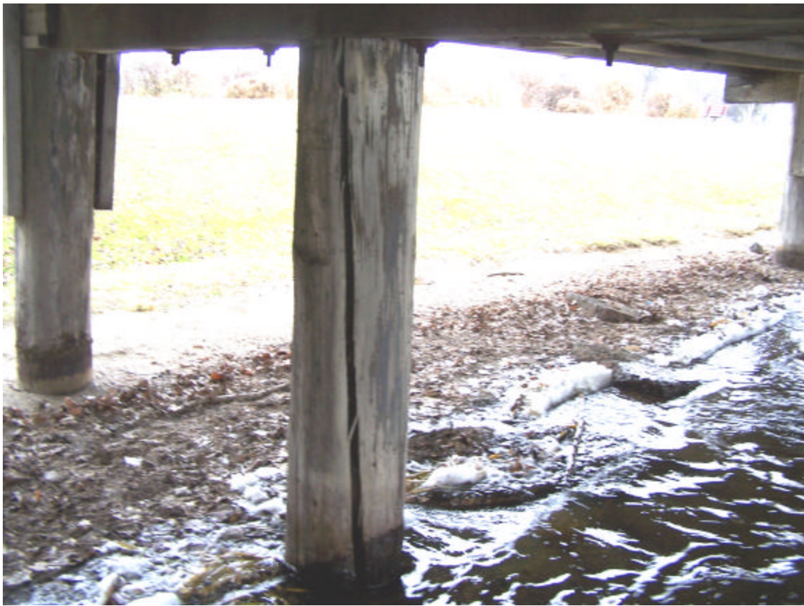
Photo 3 – Pile (severe splitting)
