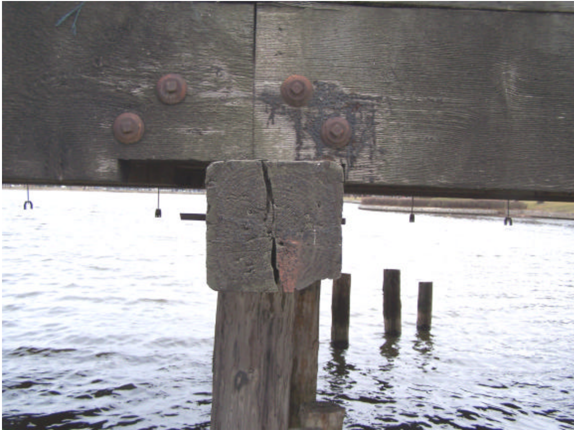
Photo 14 – Pile cap (minor splitting)
