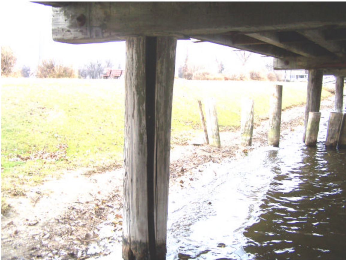
Photo 5 – Pile (severe splitting)
