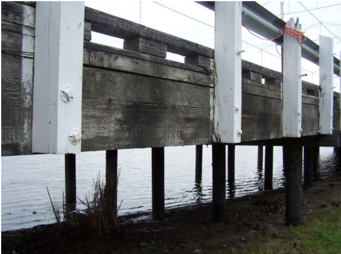
Photo 26 – Stringer (severe splitting)
