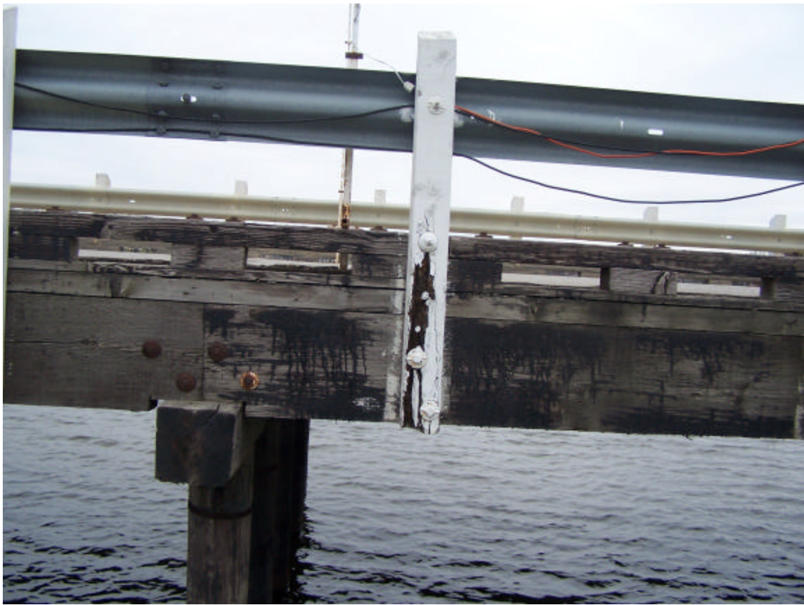
Photo 27 – Handrail post damage
