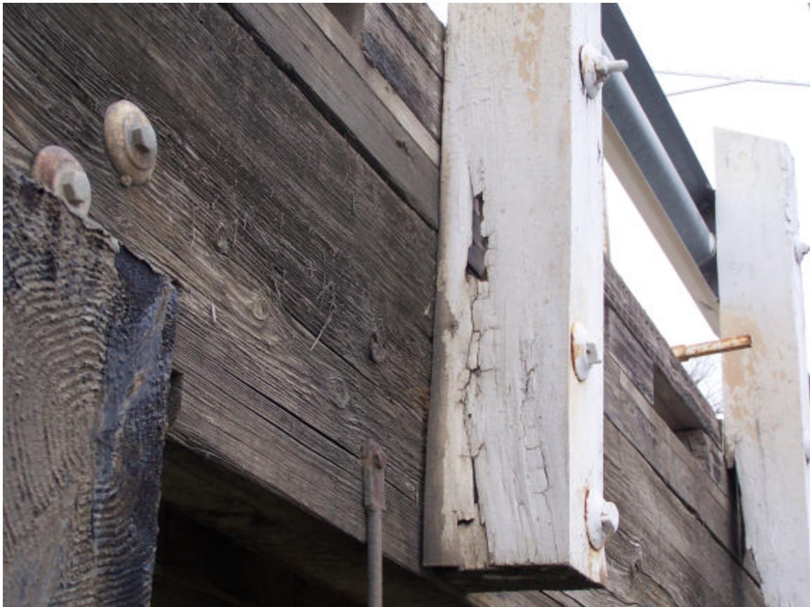
Photo 30 – Handrail post damage
