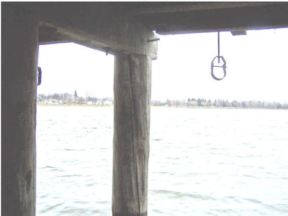
Photo 6 – Pile (minor splitting)
