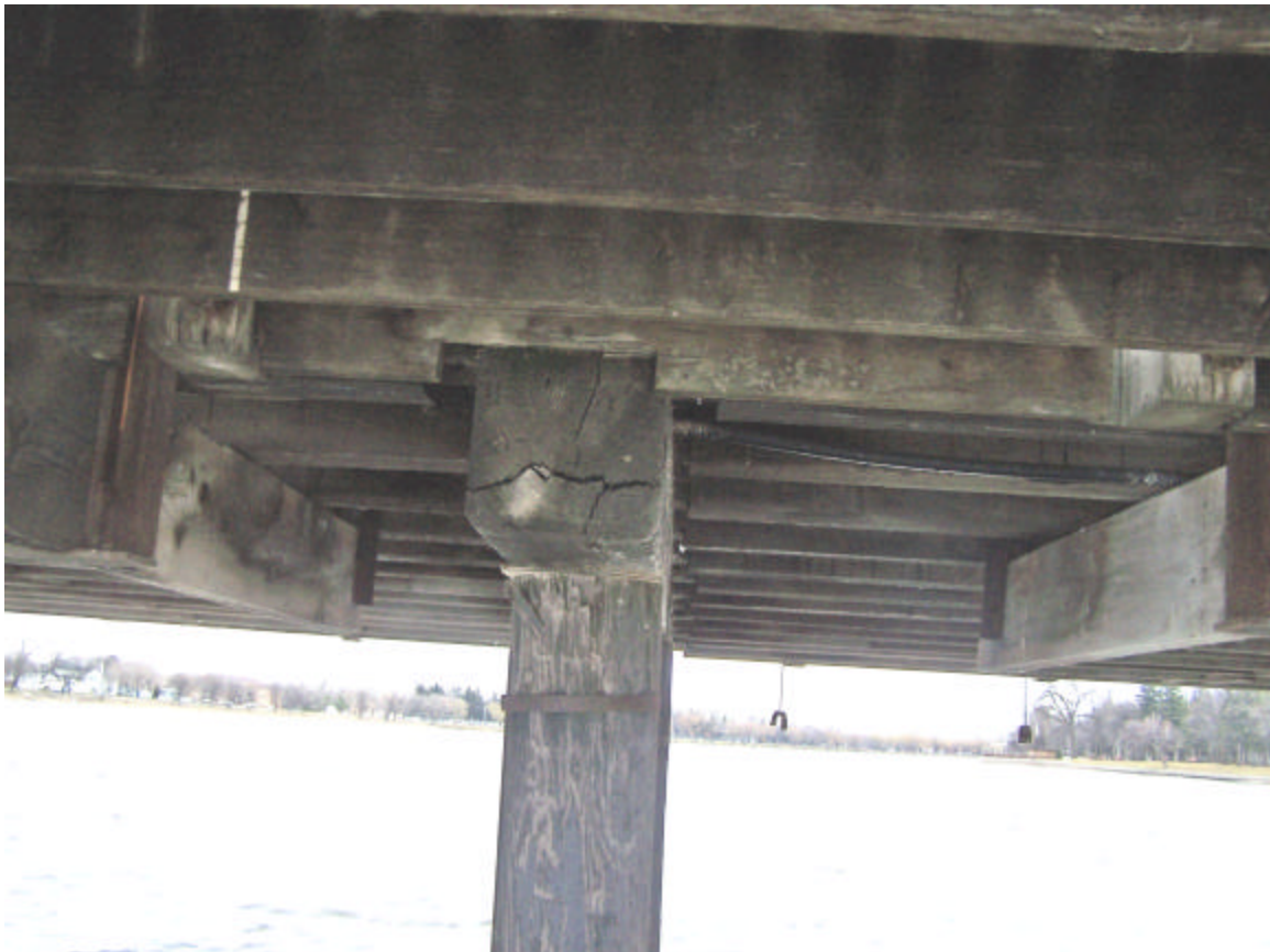
Photo 16 – Pile cap (minor splitting)
