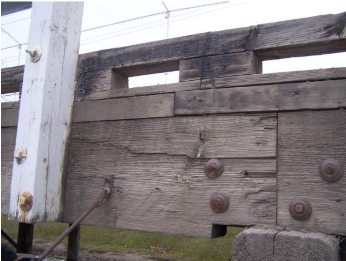
Photo 19 – Stringer (minor splitting)
