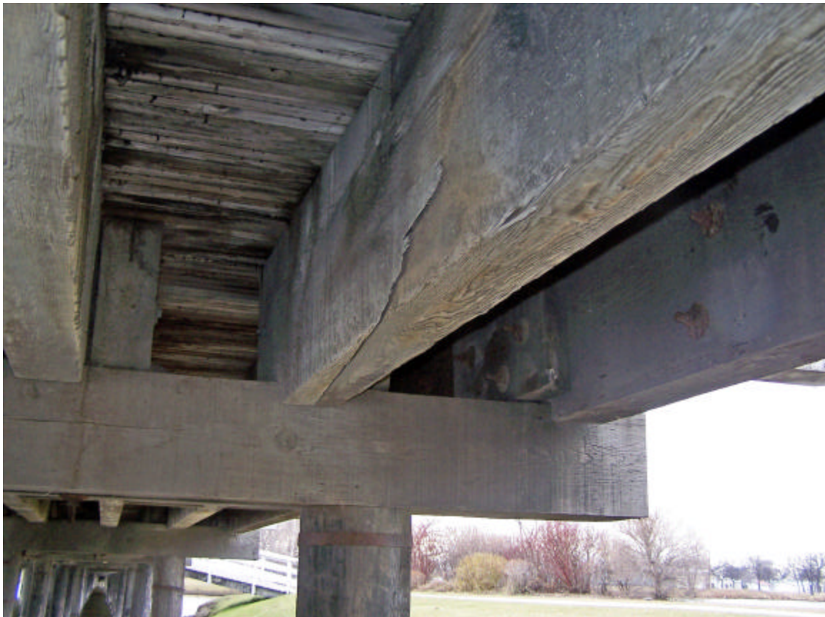
Photo 24 – Stringer (severe splitting)
