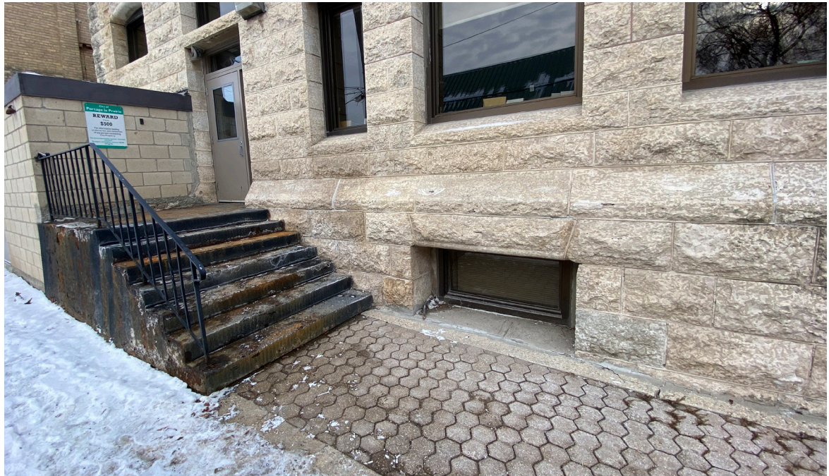
Fig. 8 Rear Entrance; recommend replacement with entrance ramp
