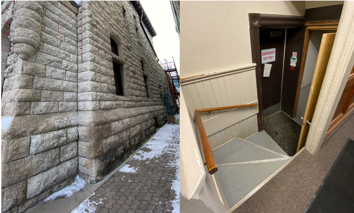
Fig. 9 Side Entrance; recommend providing ramp access up to main floor level
