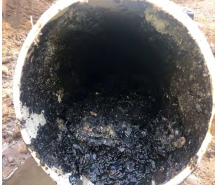
Build up in pipe
